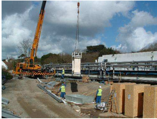
Membrane cassette being prepared at St Saviours Water Treatment Works
